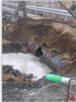
Sewer Main Breaks
