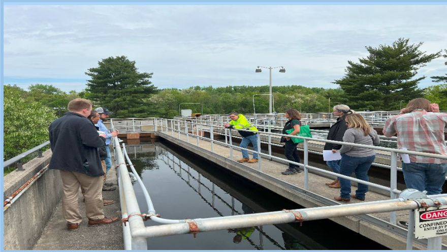
***Flocculation basin at the Burlington City Water Plant. Photo by Paul Britt of NJ Water Association***
